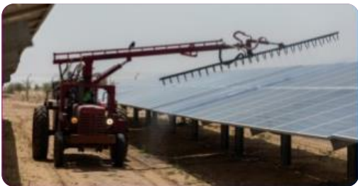
Innovation in Module Cleaning System (Semi - Automatic)
