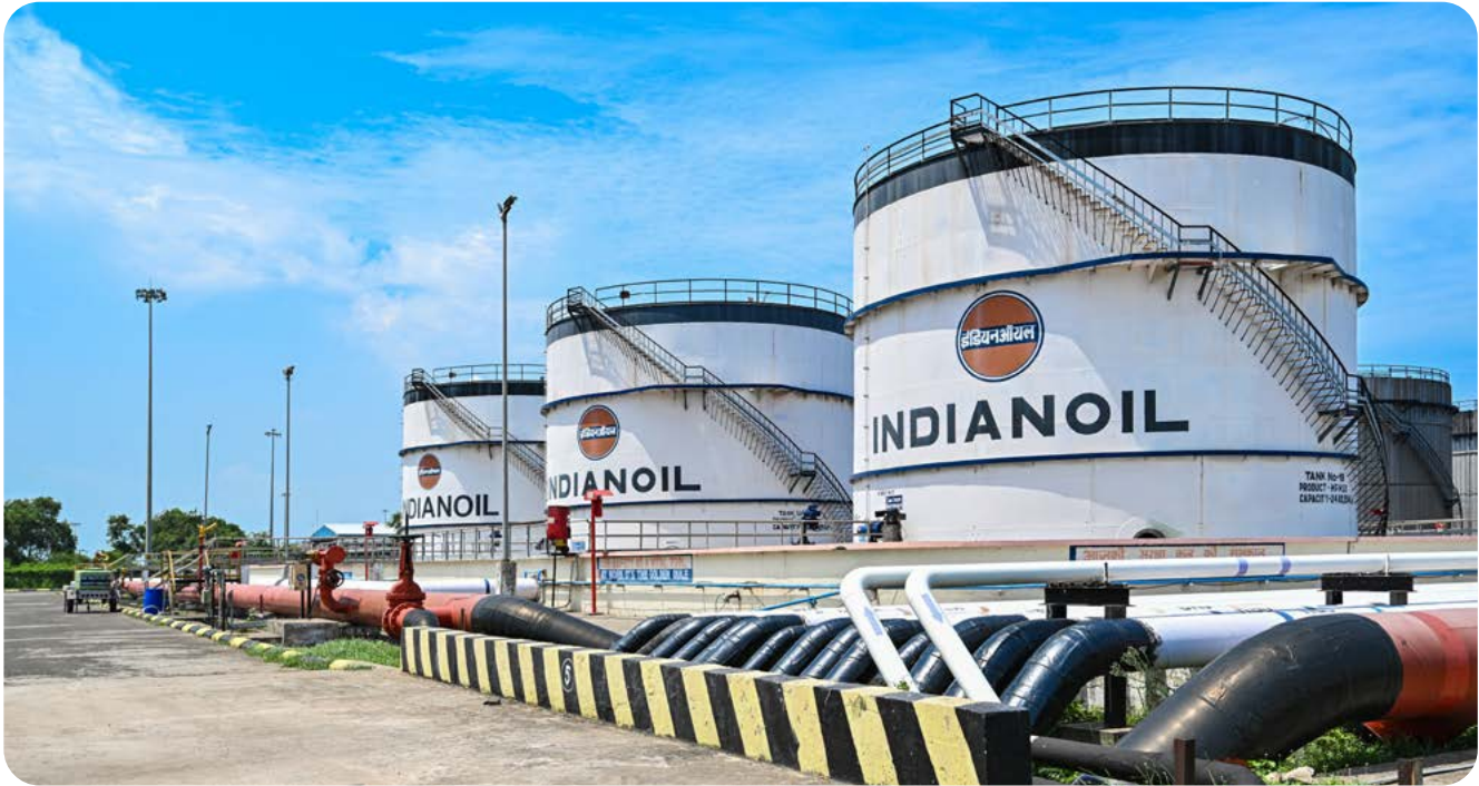
Paradip Marketing Terminal Tank Farm supporting the seamless distribution of energy across eastern India
