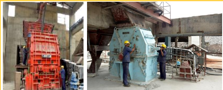
Primary and Secondary Crusher
