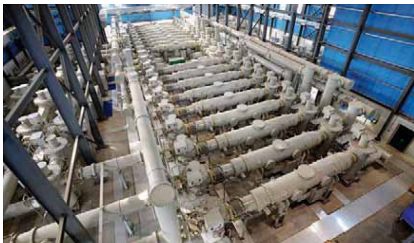
India's first 765 kV Gas-insulated Substation, at Pune.
