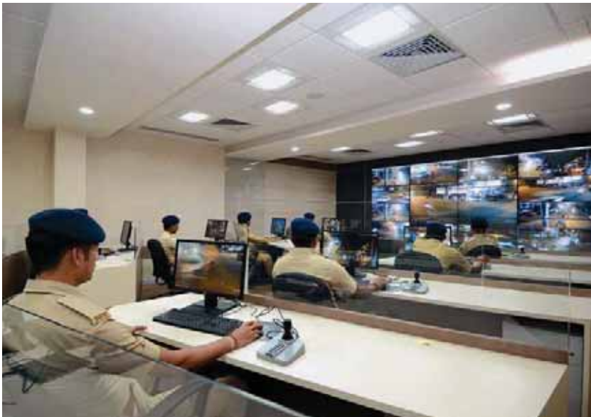
High-technology surveillance systems ensure 24x7 security.
