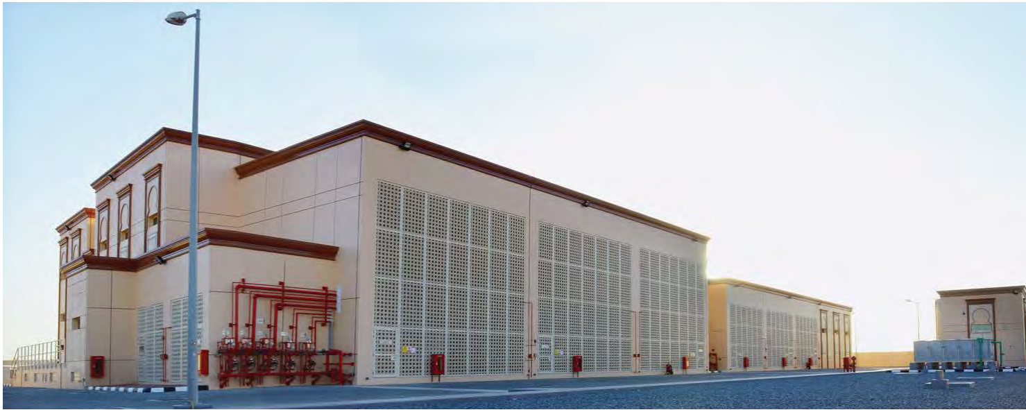
132/33/11kV Substation, Umm Al Quawain, UAE
