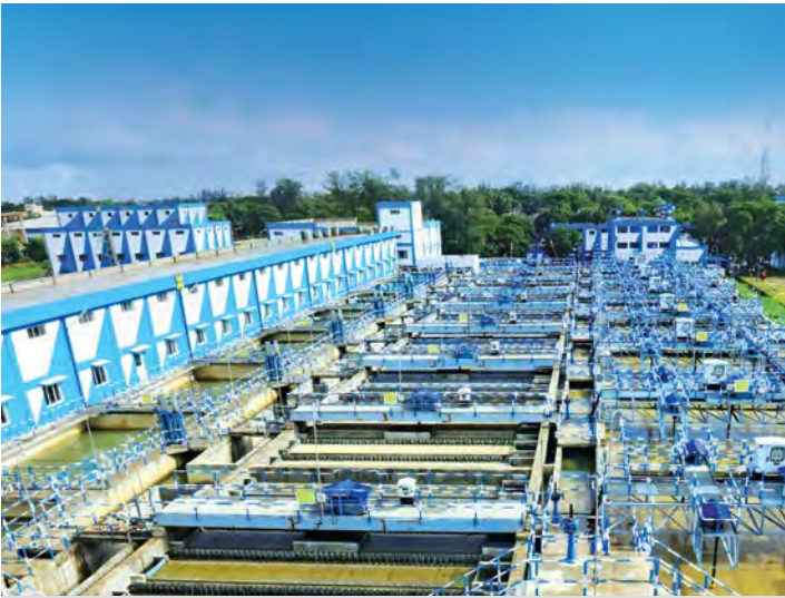
227 MLD Water Treatment Plant, Kolkata, West Bengal
