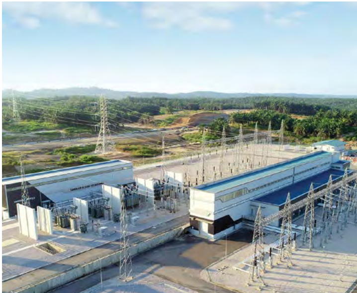
275/132/33kV Gas Insulated Substation, Samalaju, Malaysia
