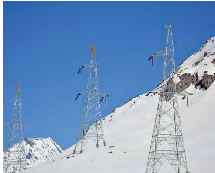
220 kV Alusteng-Drass Transmission Line, Jammu
