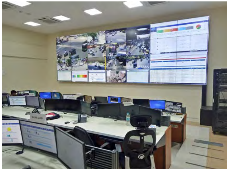
City Command & Control Centre, Vadodara Municipal Corporation.
