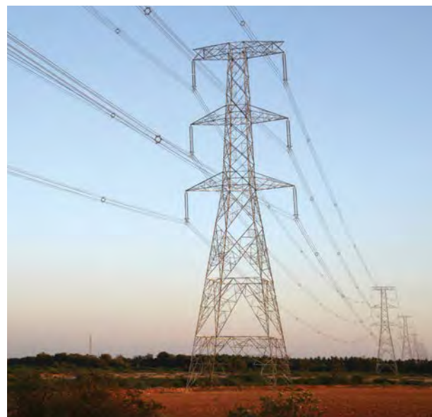
765 kV DC Kudgi Transmission Line project
