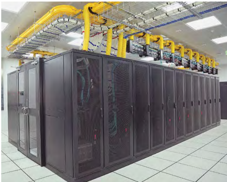
Data Center, Hyderabad
