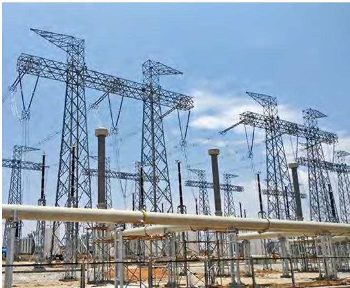
765 kV Gas Insulated Substation, Hyderabad
