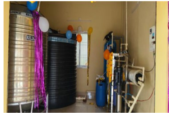
RO water plant
