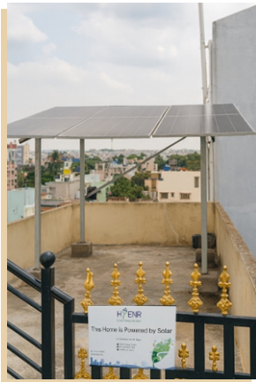
Kengeri, Bangalore | 3KWp
