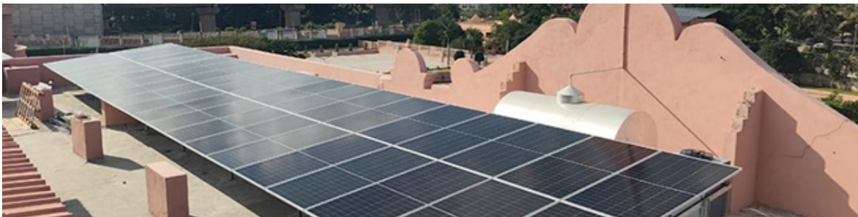
200 KWp at Karnataka
