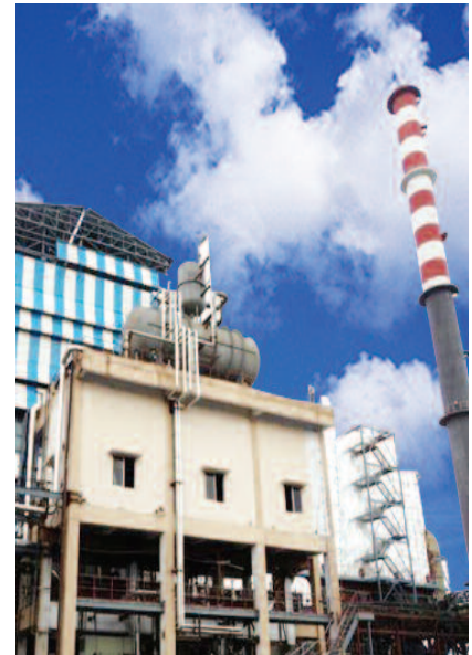
125 TPH Power Boiler No.6
