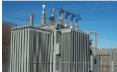
Transformer & Sp Oil
