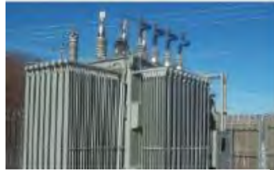
Transformer & Sp Oil
