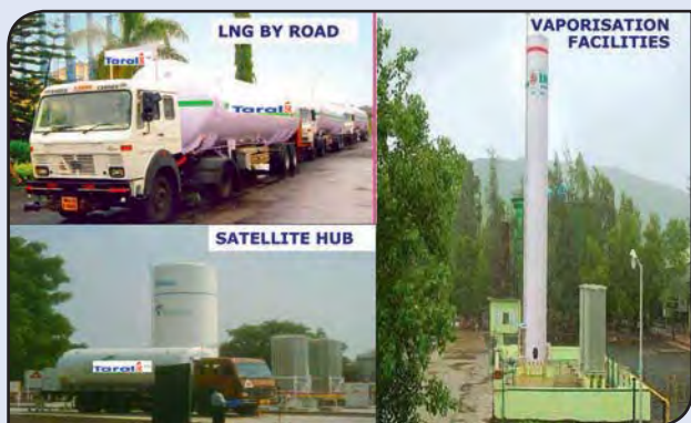
Facilities for Supply of LNG by Road
