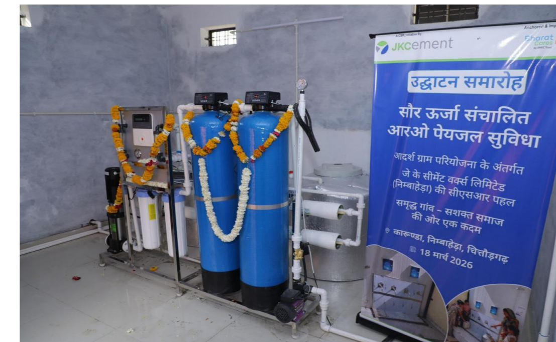
Solar RO Installation at Nimbaheera
