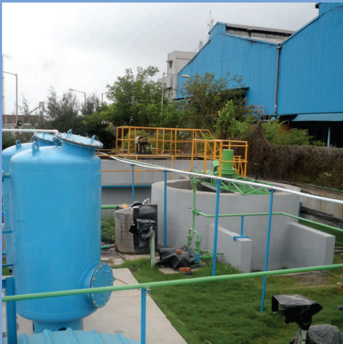
Sewage Treatment Plant - Moraiya Unit
