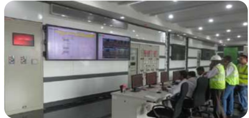
Central control room
