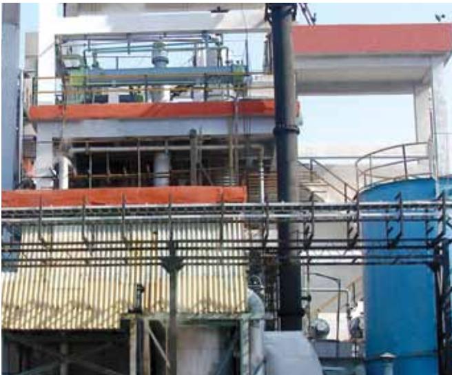
New membrane plant
