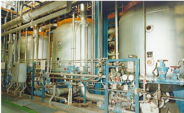
CPP – Condensate Polishing Plant
