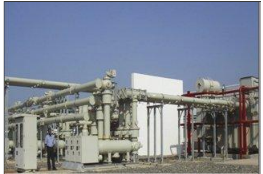
230/11 KV Gas Insulated Substations, Hyundai, Chennai
