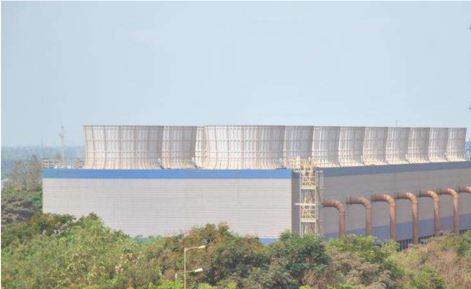
IDCT – Cooling towers
