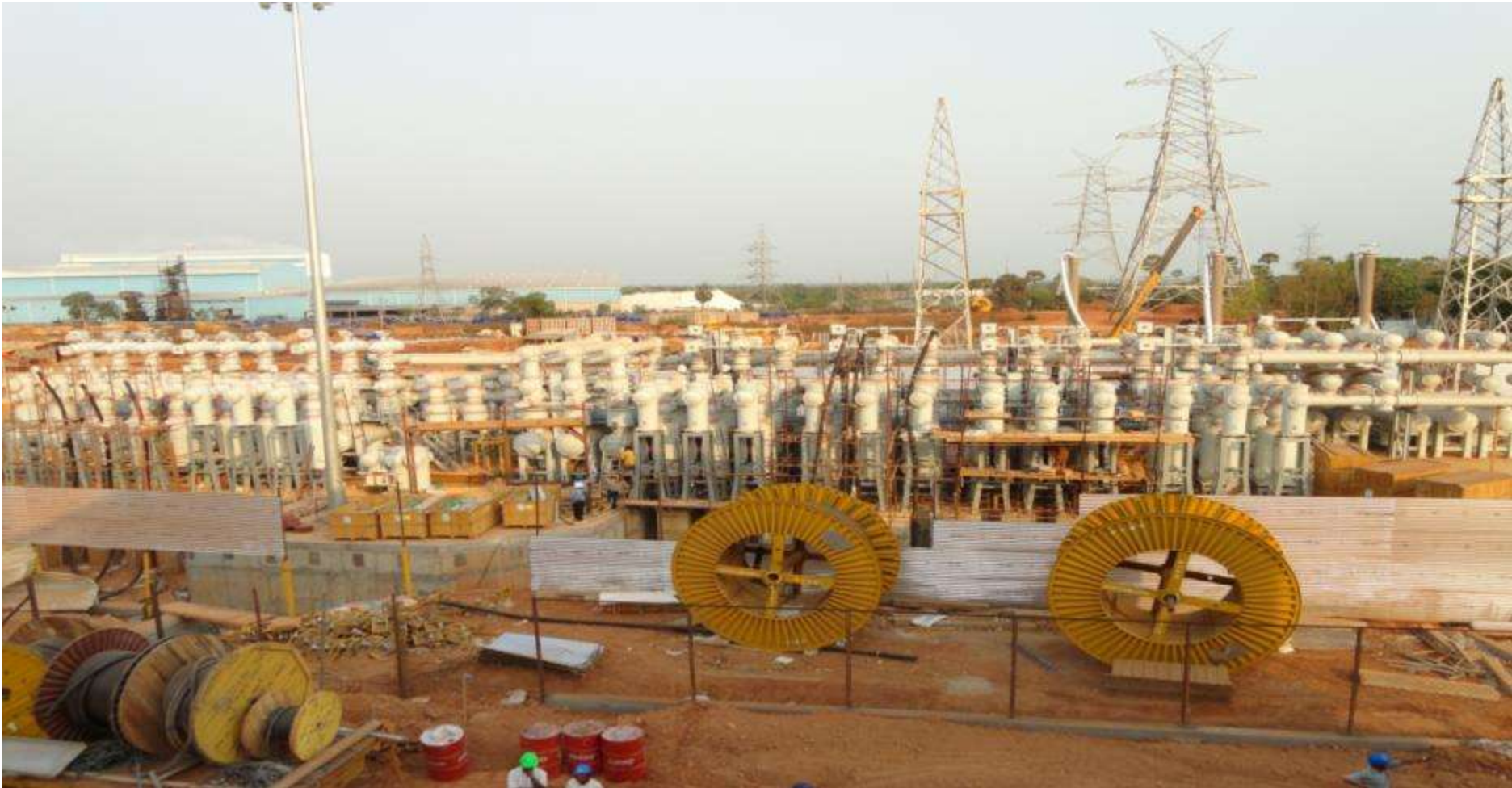
Gas Insulated Switchyard and Transmission Towers
