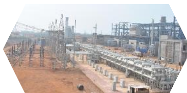
Samalkot Power 2,400 MW
