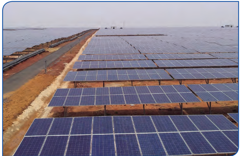
500 MW Solar PV plant of APGENCO in Andhra Pradesh financed by REC.
