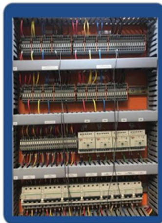
Power Distribution Industrial Panel
