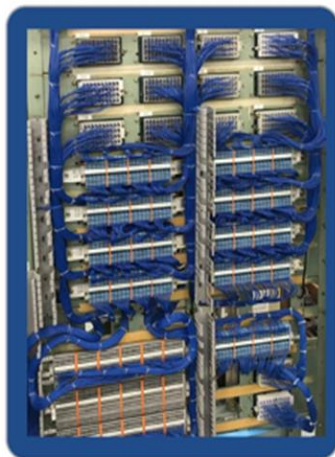
Railway Signalling Panel
