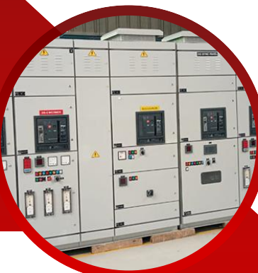
Control Panels & Distribution Panels
