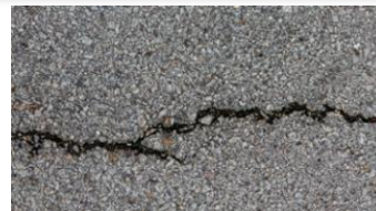
Pavement distress identification
