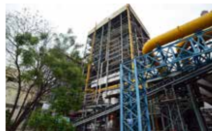
View of Boiler, Vijayanagar
