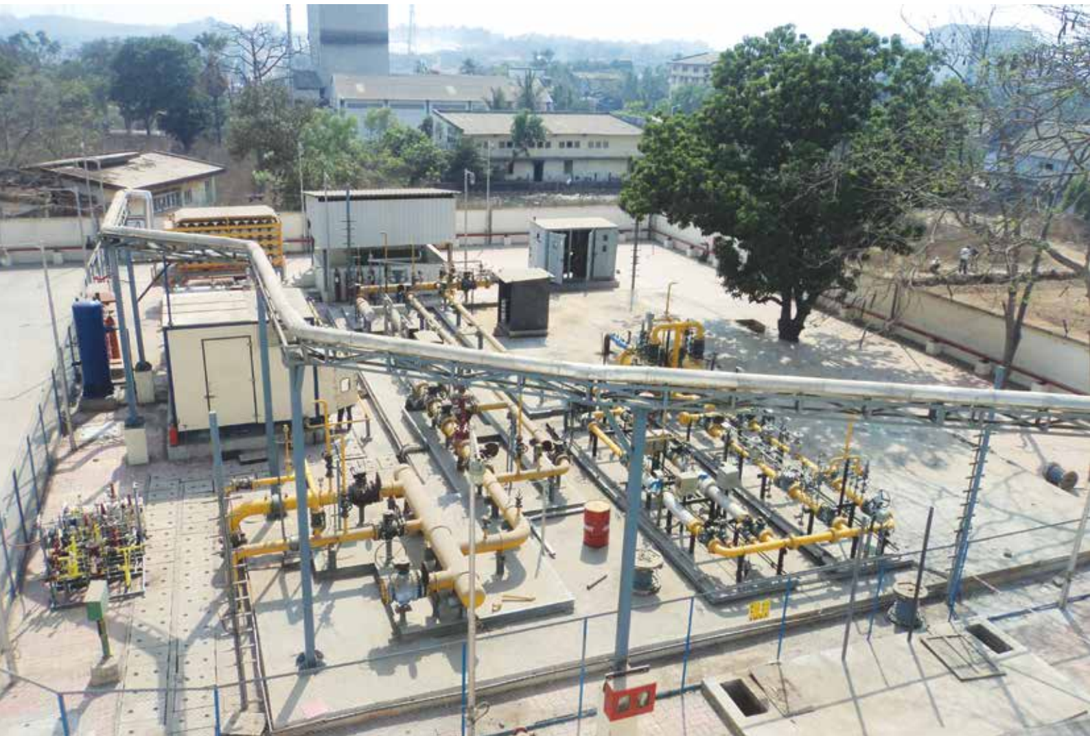
City Gate Station, Mahape.
