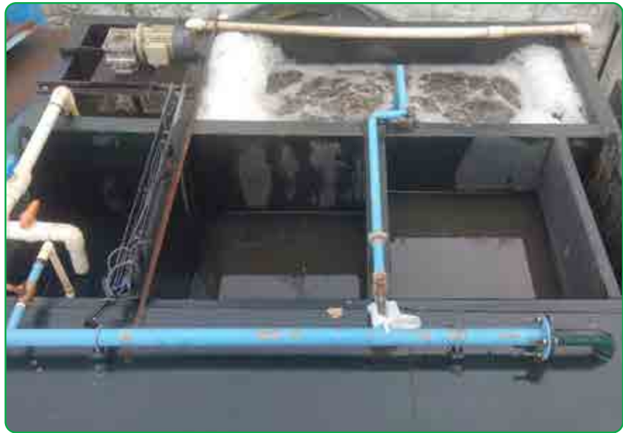
➤ Sewage Treatment Plant installed at CGS Mahape
