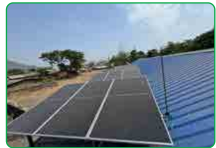
➤ Solar Off-Grid System installed in Villages of Raigad
