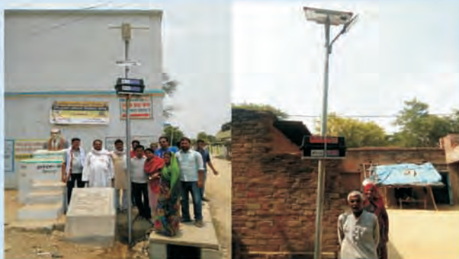
Solar Street Lighting System
