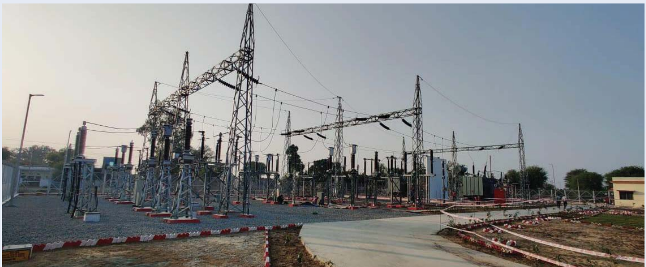
132/25 kV traction sub-station at Banasthali Newai, Jaipur- Sawaimadhopur Section, NWR
