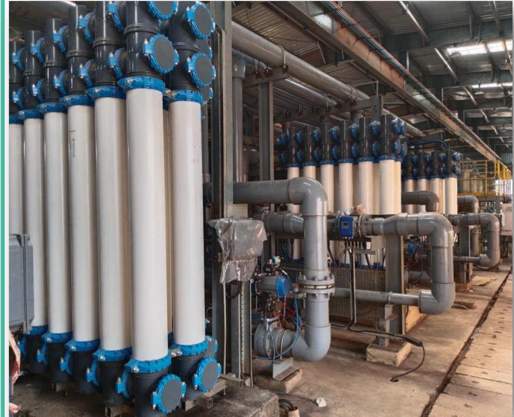
NMDC ZLD Plant, Chhattisgarh, India
