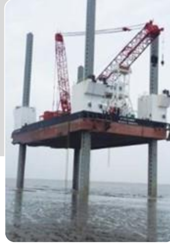
8 Large-capacity Jack ups (200–750 tonne)
