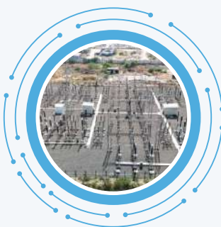
66 kV Power arrangement at GIDC saykha (Private)
