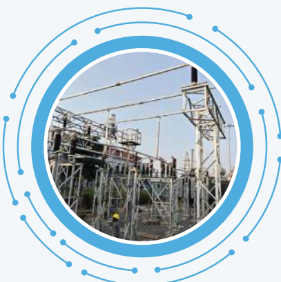
400 kV & 66 kV CIS Substation, Bhogat (Dwarka)
