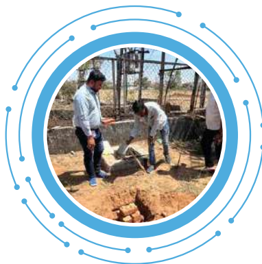
TN-119 Substation Project- Pratapnagar, Jaipur (Government)
