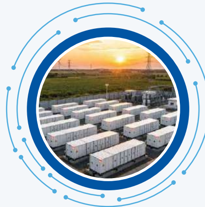
Battery Energy Storage System Project 65 MW/130 MWh-Gujarat
