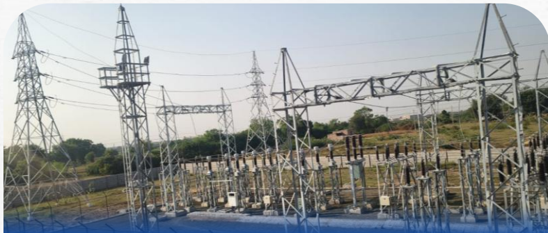
66 kV Switchyard for 30 MW Solar power plant (Private)
