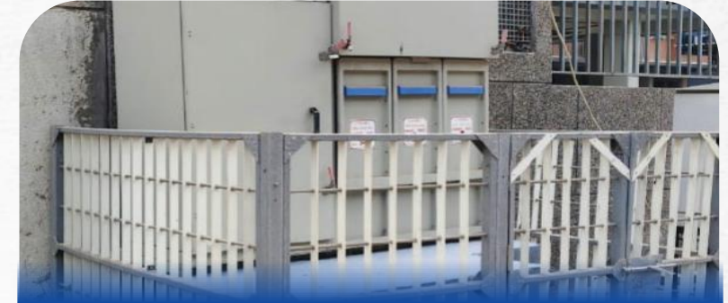
RDSS Scheme commissioned at Gandhinagar for UGVCL (Government)
