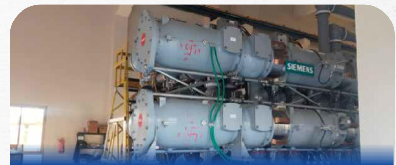
220KV GIS Bay Equipment - Atul GIS SS (GETCO) (Government)
