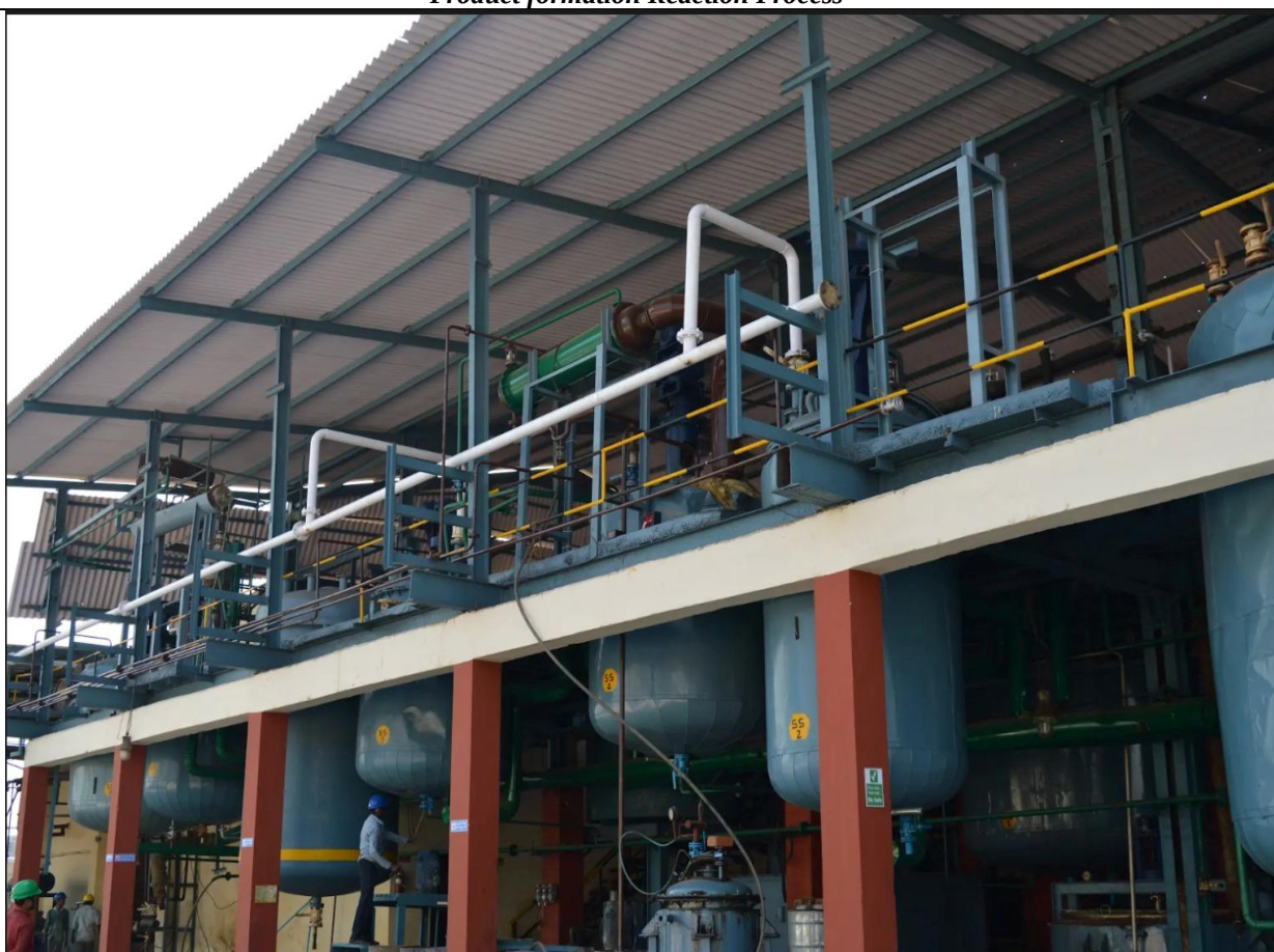
Reactors in Plant 3
