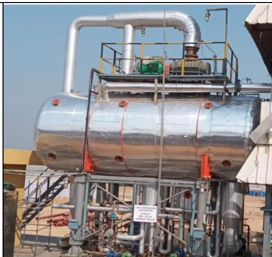
MVR_ waste water treatment facility
