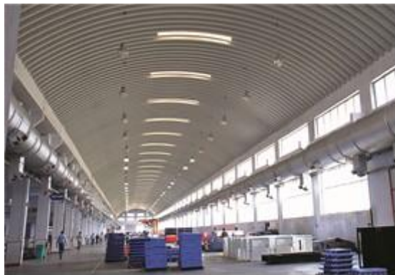
Roof with Hanging Ducts
