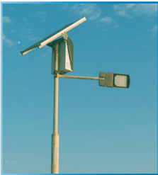
Solar Street Light
