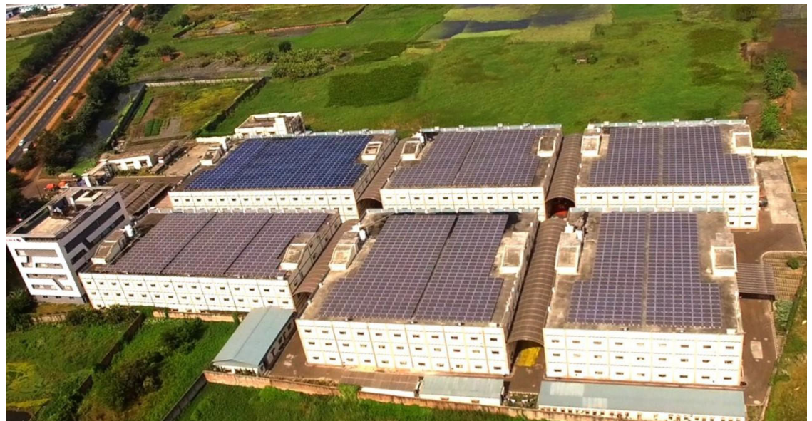
Rooftop solar power plant at Dankuni unit
