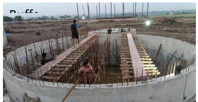
Buffer Tank (Ariel View)
