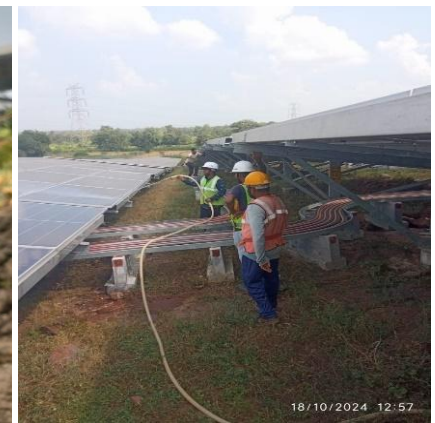
Solar Module Cleaning
