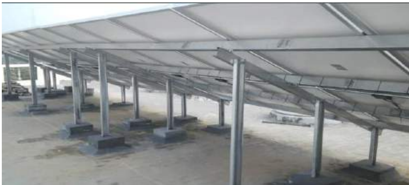
Solar panel mounting structures
