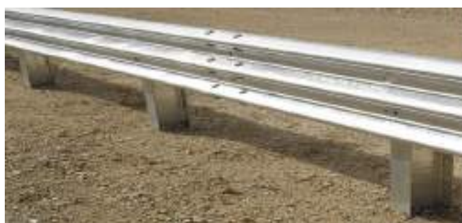
Thrie Beam Guardrail
