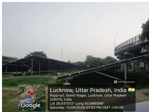
Ground-Mounted Solar Plant, Gomti Nagar, Lucknow
