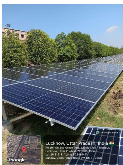
Ground-Mounted Solar Plant, Lucknow, Uttar Pradesh
