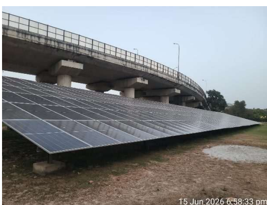
Ground-Mounted Solar Plant
