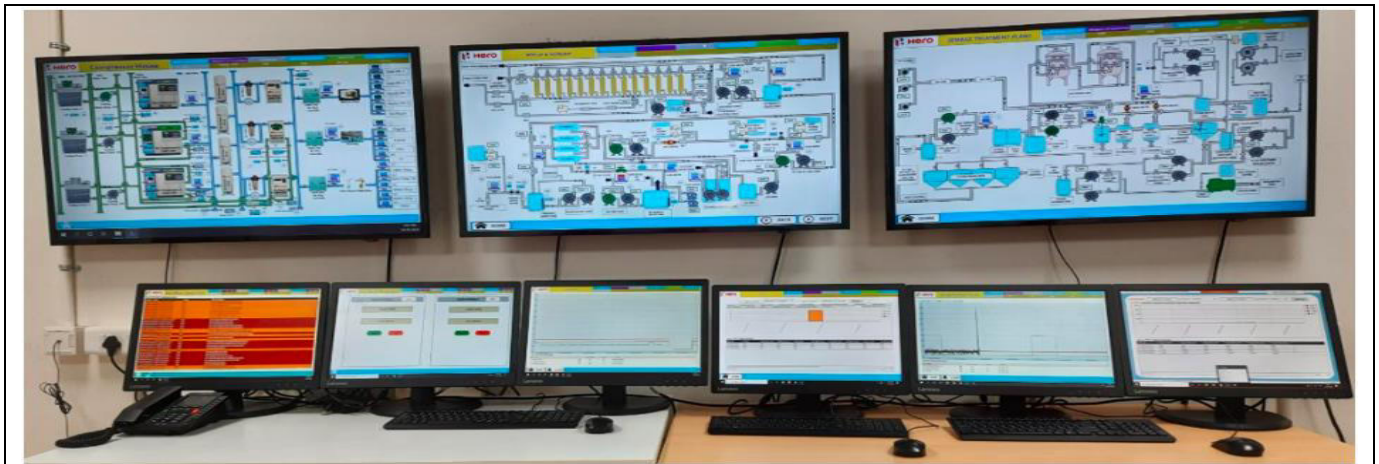
Utility Monitoring & Controlling Systems
