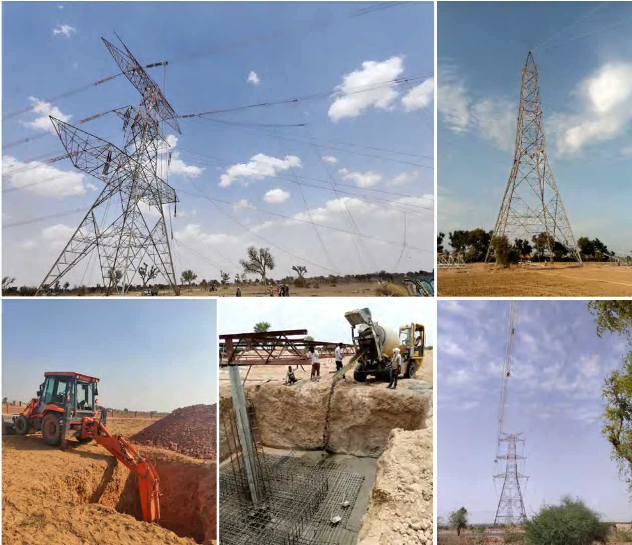
Project 765kV Fatehgarh 2 to Bhadla 2
