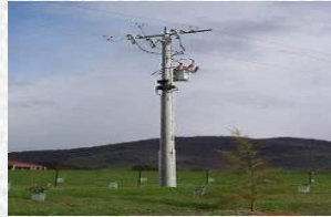
Power Distribution Poles
