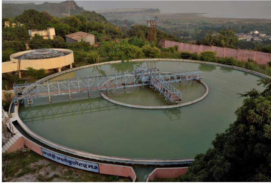
Fig. 55-Water Treatment Plant in NCL
