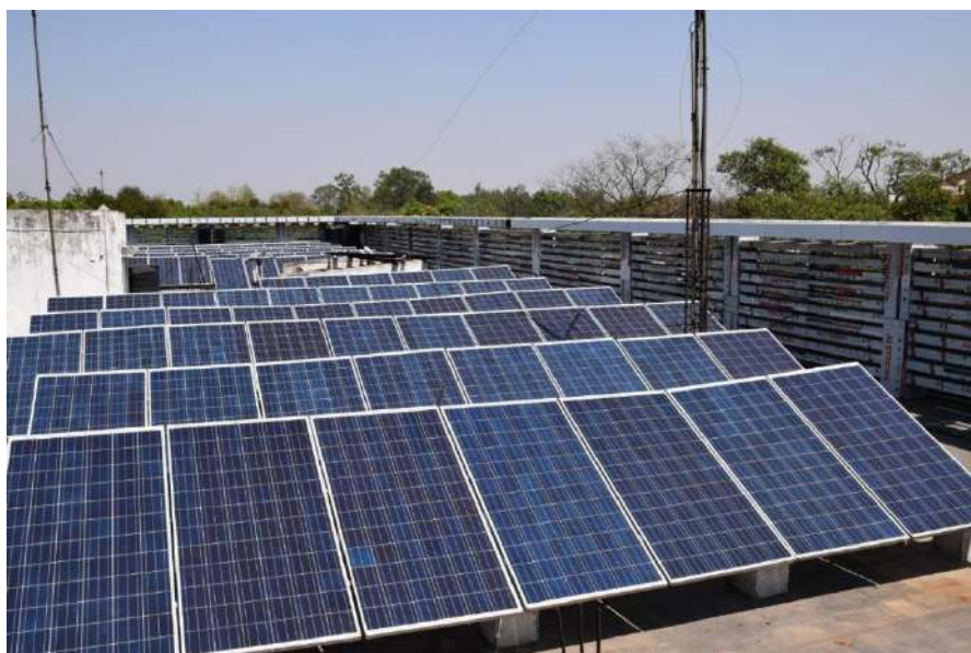
Fig. 70- Roof top Solar plant at CCL
