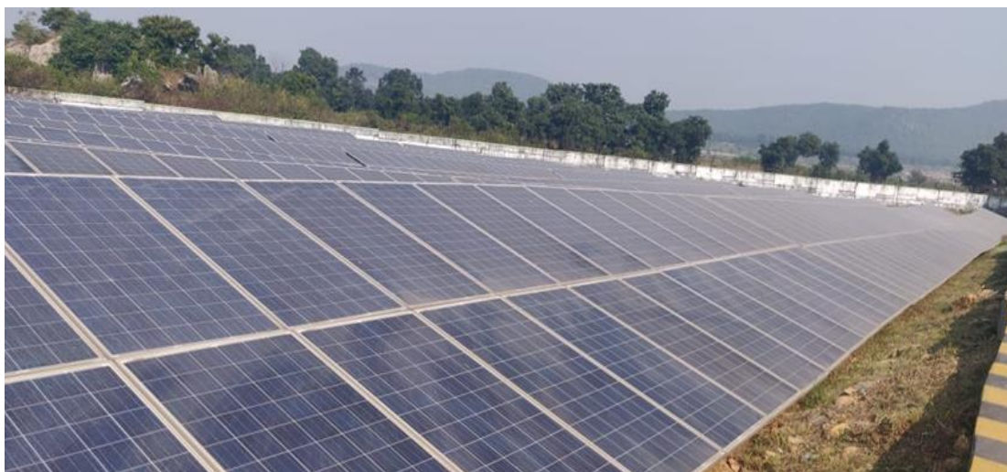
Fig. 67 - Ground mounted Solar Power Project of MCL
