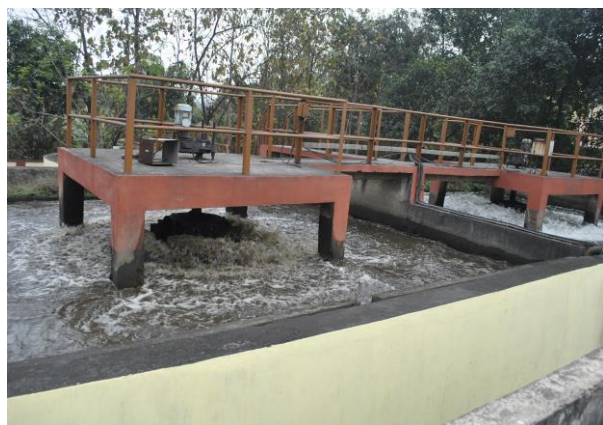
Fig. 50 - STP in Ananta OCP of MCL
