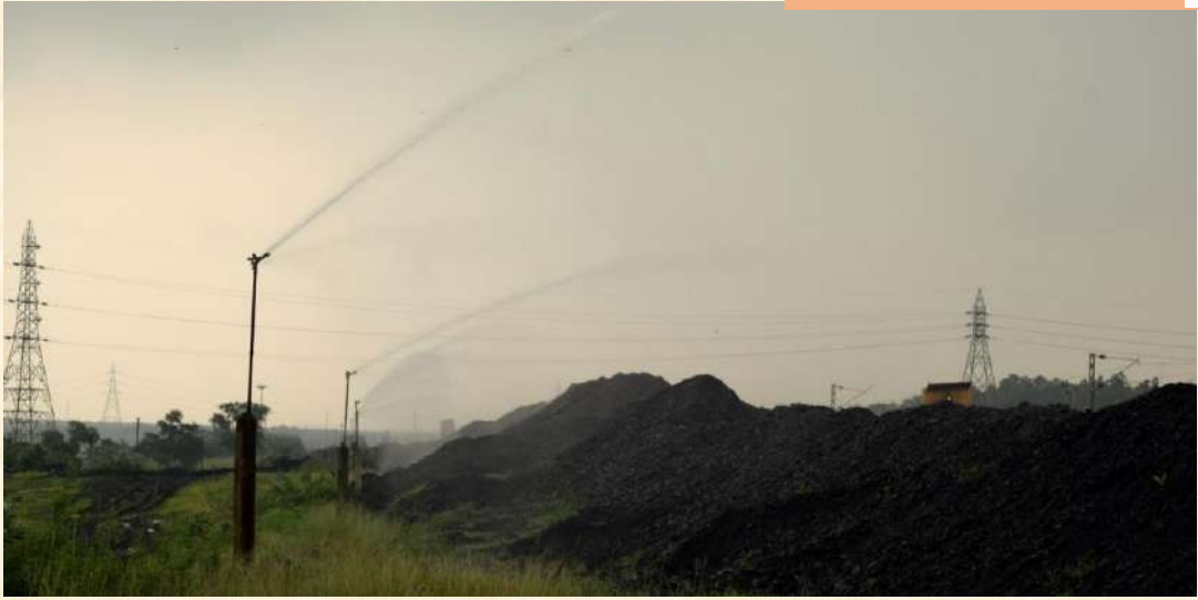
Fig. 46 - Fixed Sprinkler in Belpahad OC, MCL
