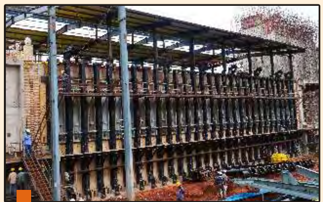
Coke Oven Battery
