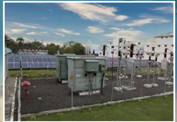
1.7 MW Solar PV plant at Bina, Madhya Pradesh for Indian Railways
