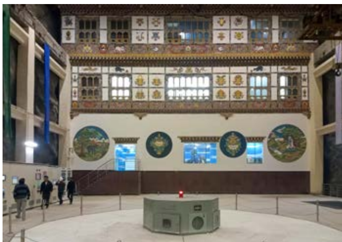
Turbine hall of 4x180 MW Mangdechhu HEP project in Bhutan
