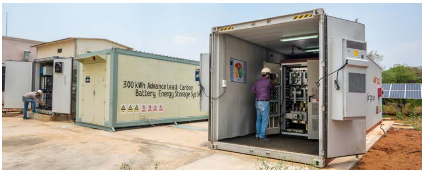
1MW Battery Energy Storage System (BESS) for in-house usage, developed & commissioned at Corporate R&D, Hyderabad
