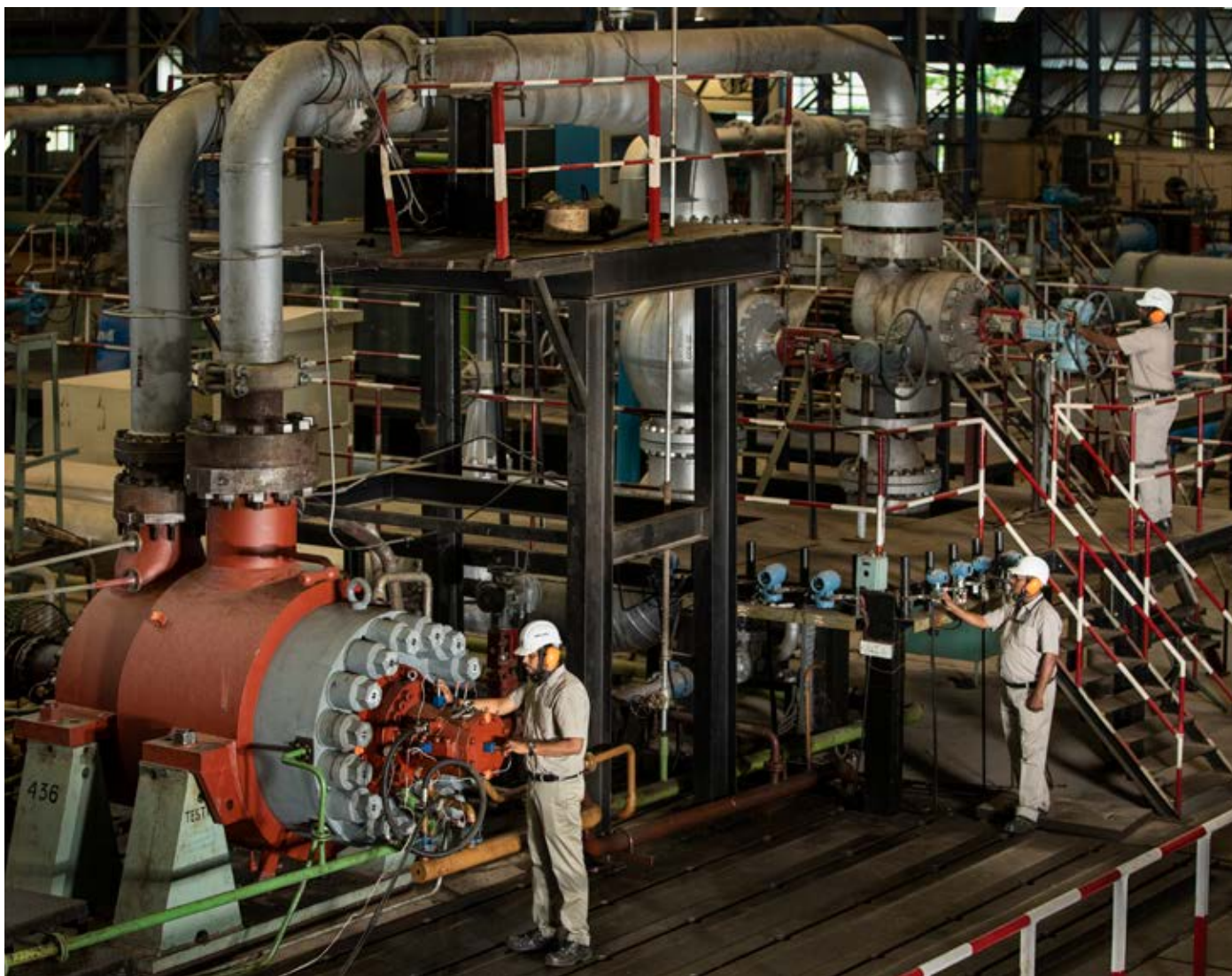
Simulation studies being carried out on BHEL power equipment at HPEP Hyderabad
