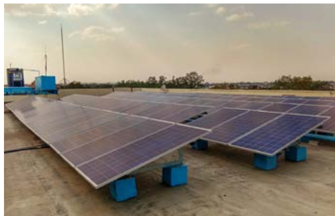
295 kW p in-house developed Solar Rooftop SPV panel at BHEL Bhopal
