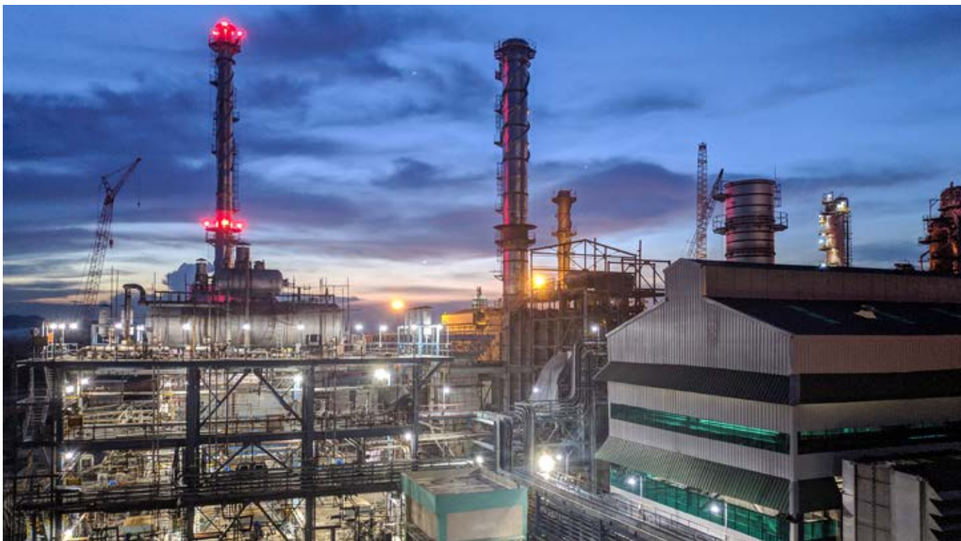
RFCL Ramagundam CPP with 32.5 MW rating Gas Turbine along with Utility Boiler and Heat Recovery Steam Generator - under commissioning by BHEL in Telangana
