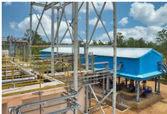
2.0 MLD capacity Sewage Treatment Plant (STP) at BHEL Tiruchirappalli
