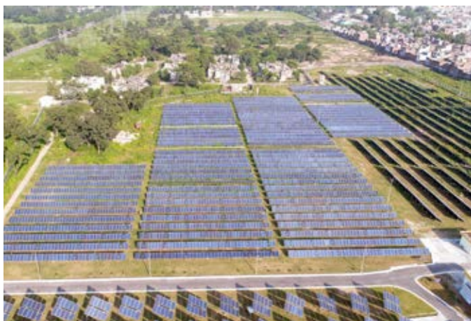
5 MW solar power plant including ground mounted, fixed, motor tracking & passive tracking enabled modules of BHEL make at Haridwar plant premises
