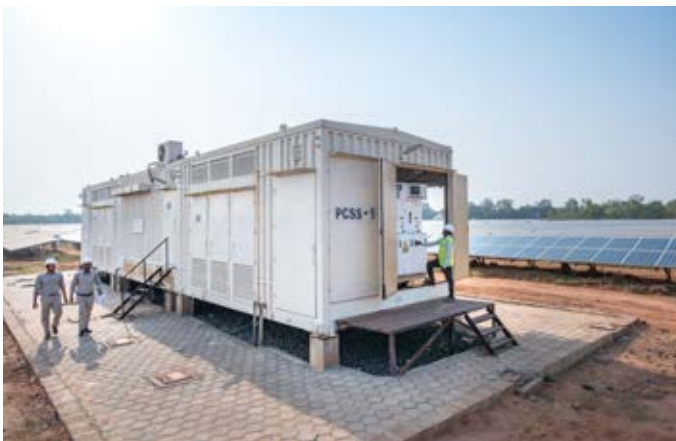
Battery Energy Storage System (BESS) integration at 65 MW SPV plant at Neyveli, Tamil Nadu, commissioned by BHEL
