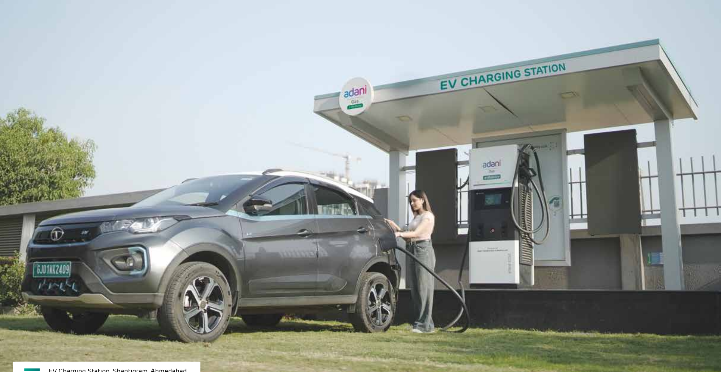
EV Charging Station, Shantigram, Ahmedabad
