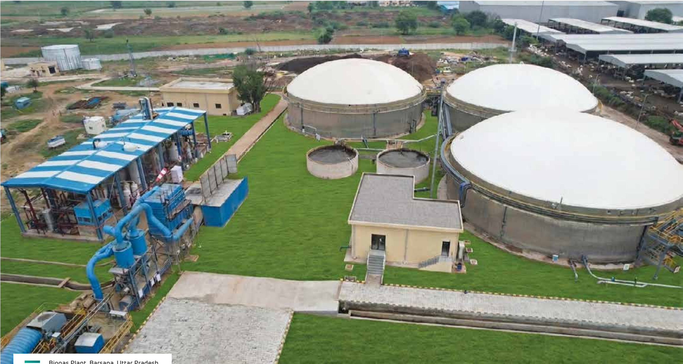
Biogas Plant, Barsana, Uttar Pradesh
