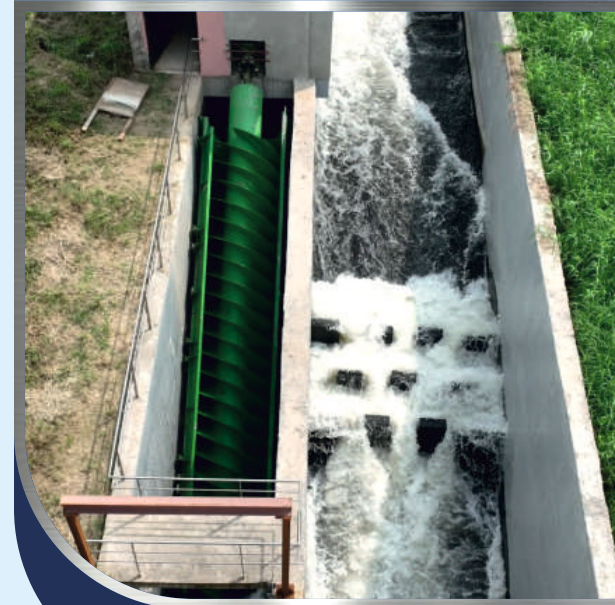
40 MGD Rithala STP - Delhi
